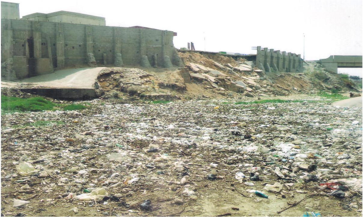
Plate 6. Dilapidated embankment along the riverbank.
