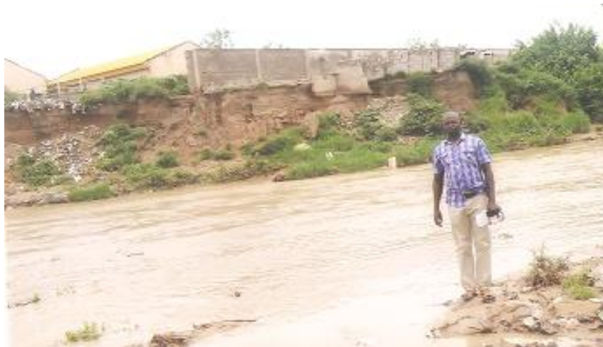
Plate 2. Mass wasting adjacent a construction company.
