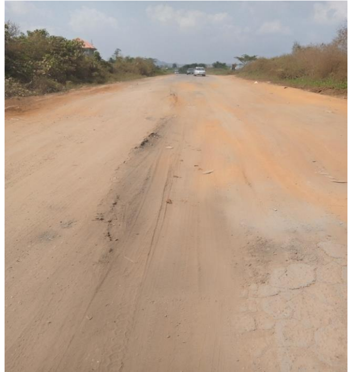
Plate 1. Failed Segment at location 1 before its recent reconstruction/rehabilitation.
