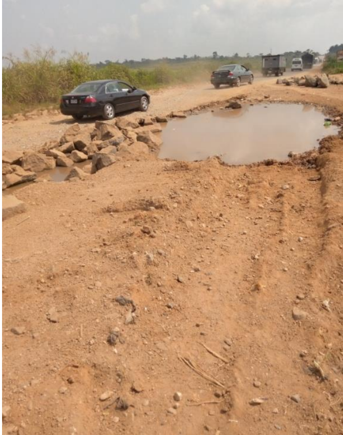
Plate 2. Failed Segment at location 2 before its recent reconstruction/rehabilitation.
